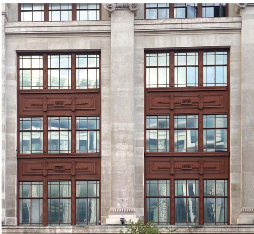
M&S's flagship building is characterised by sophisticated classical elevations, with ornate recessed oxidised window panes and decorative stonework (Credit: SAVE Britain's Heritage)
